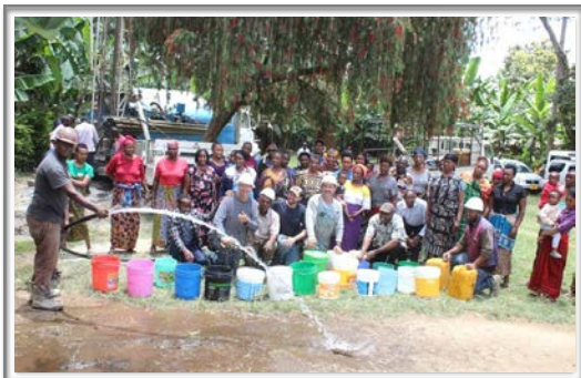
Wyoming friends drilled a new well, bringing clean water to the people of Mula village for the first time!
